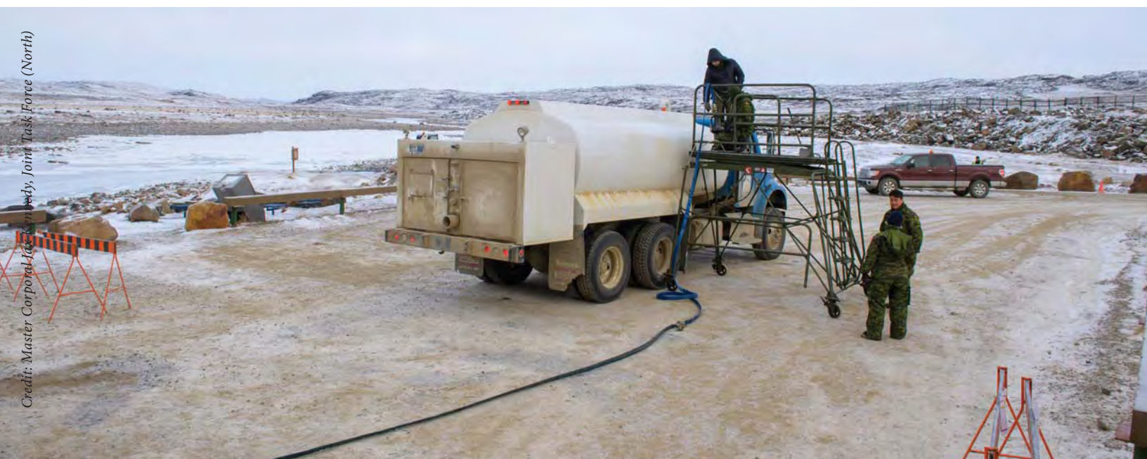
Members of 4 Engineer Support Regiment fill the first water truck with potable water produced from the Reverse Osmosis Water Purification Unit that was established during Iqaluit's water contamination crisis in November 2021.
